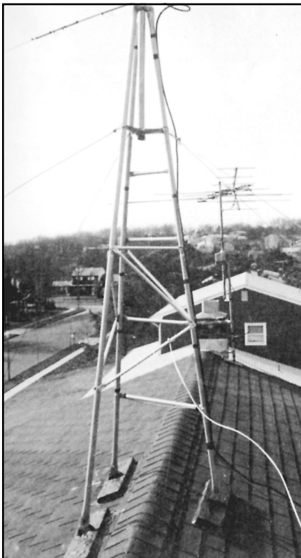
Fig 35 —This tripod tower supports a rotary beam antenna. In addition to saving yard space, a roof-mounted tower can be more economical than a ground-mounted tower. A ground lead fastened to the lower part of the frame is for lightning protection. The rotator control cable and the coaxial line are dressed along two of the legs. (Photo courtesy of Jane Wolfert)
