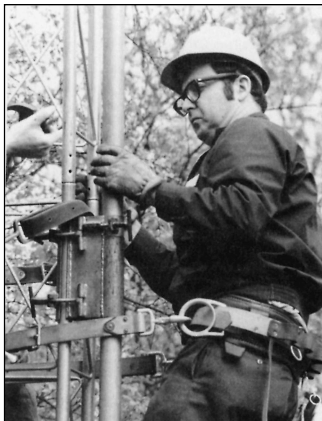
Fig 1—Bill Lowry, W1VV, uses a good quality safety belt, a requirement for working on a tower. The belt should contain large steel loops for the snap straps. Leather loops at the rear of the belt are handy for holding tools. (photo by K1WA)
