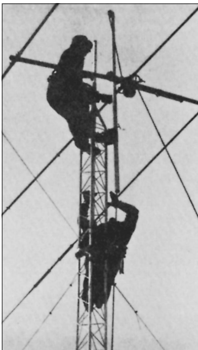
Fig 20—A gin pole is helpful in positioning antennas and tower sections. The weight of the assembly is held by the ground crew via a heavy rope, making tower work safer and less tiring. (Photo by Dave Pietraszewski, K1WA)
