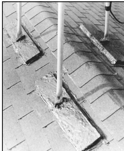
Fig 37 —Three lengths of 2 \times 6 wood mounted on the outside of the roof and reinforced under the roof by three identical lengths provide a durable method for anchoring the tripod. A thick coat of roofing tar protects against weathering and leaks.
