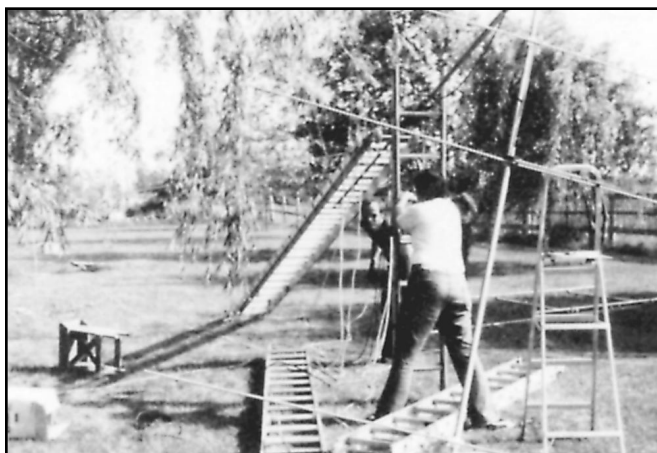
Fig 6 —Walking the ladder up to its vertical position. Keith, VE2AQU, supports the mast with a second ladder while Chris, VE2FRJ, checks the ropes. (Photo by Keith Baker, VE2XL)
