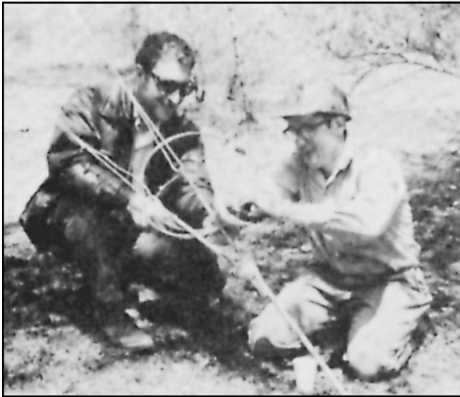
Fig 22 —A length of guy cable is used to assure that the turnbuckles remain in place after they are tightened. This procedure is an absolute requirement in guyed tower systems. (Photo by K1WA)
