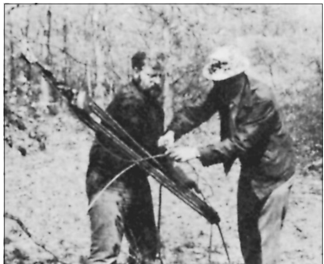
Fig 21—Proper tension can be placed on the guy wires with the aid of a block-and-tackle system. (Photo by K1WA)
