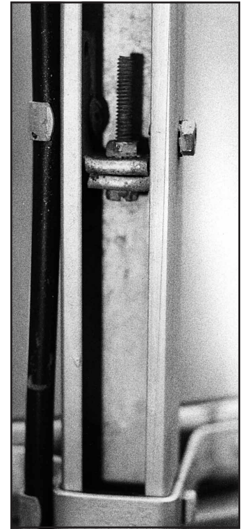
Fig 13—In this photo the open edges of the Unistrut channel are facing the viewer. The locking pin is visible in the middle of the channel.
