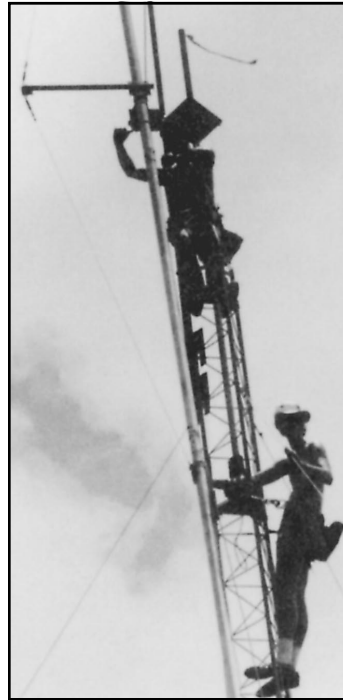
Fig 32—Working at the 70-foot level. A gin pole makes pulling up and mounting the boom to the boom plate a safe and easy procedure.
