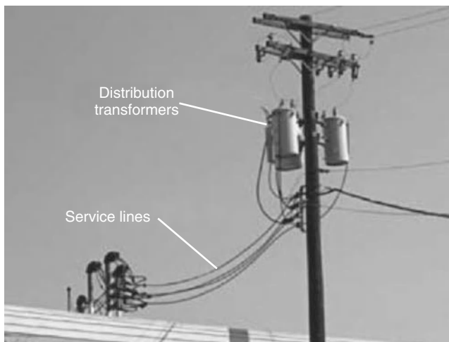
Figure 7-1. Three single-phase, pole-type transformers.
