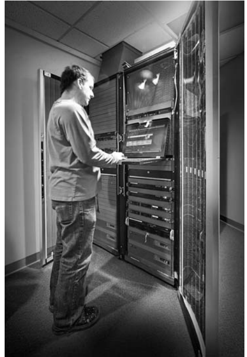
Chris Johnson at the climate-controlled computer rack, part of the HP upgrade at VATT.
